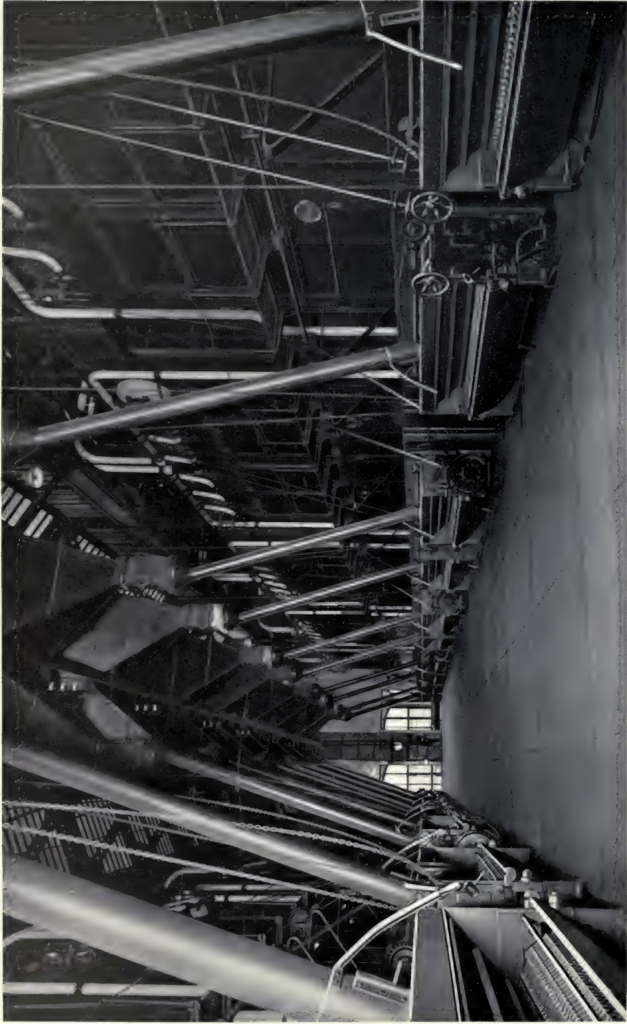
COMMONWEALTH EDISON CO., CHICAGO, ILL. NORTHWEST STATION. BABCOCK & WILCOX SUPERHEATERS INSTALLED IN 17,400 HORSE POWER OF BABCOCK & WILCOX BOILERS IN THIS STATION
